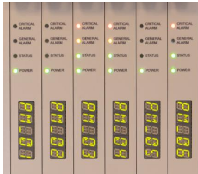
Figure 2 Critical alarm indication using LEDs on IO PCA.
